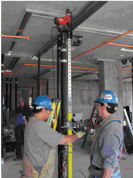
Figure 2. New inverted drill press method. The drill saddle accepts different types of drills. A switch on the column near the left hand activates the drill. The column is supported by a flat metal plate at the base.
