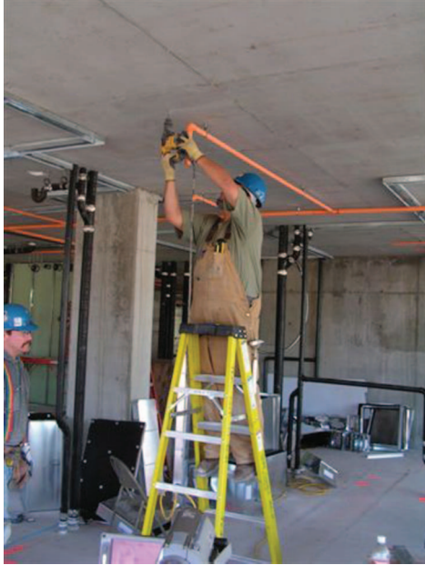
Figure 1. Construction worker demonstrating usual method of overhead drilling into concrete ceiling. The upward forces may be 20 kg-force or more. This plumber is also exposed to dust and is at risk of falling off the ladder.
