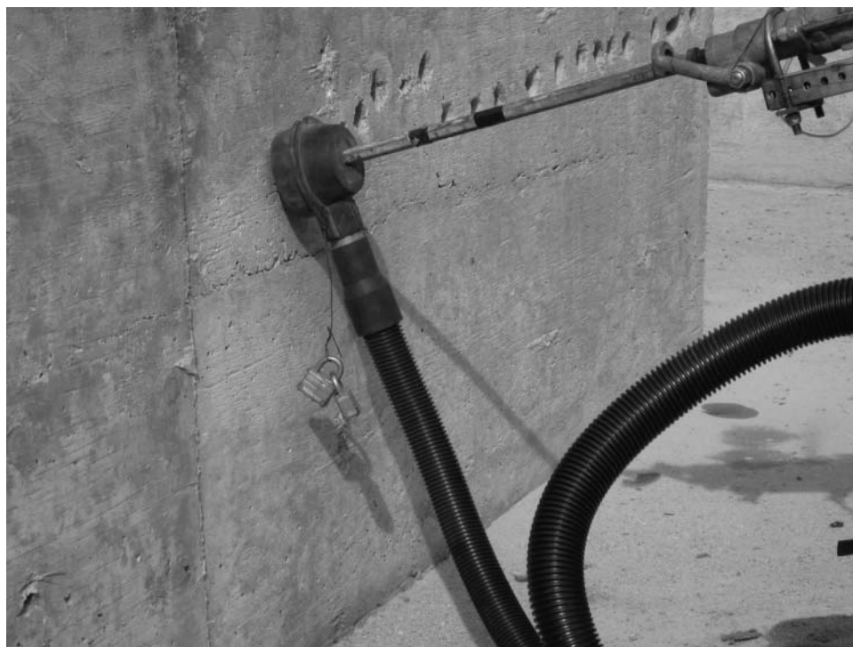
FIGURE 3. Dust capture shroud functioning while drilling. The locks were added to provide weight to the shroud so that it would slide toward the hole while drilling.
